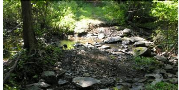
Culverts washed out on Eleanor’s Walk, carving gullies and exposing large stones in the trail bed
